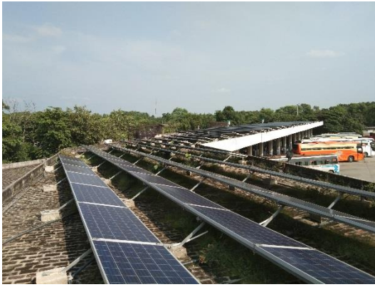
Solar Panels on roof of ISBT Building
